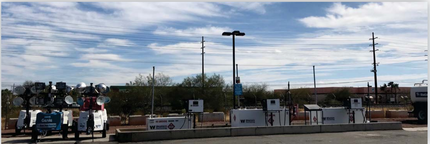
Above Ground Fueling Station and Containment System
